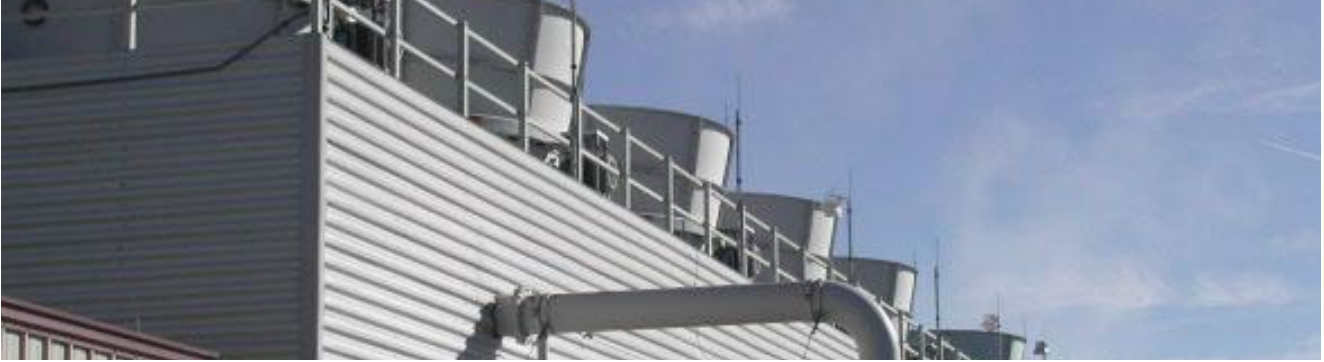
Figure 12.1 · Cooling towers are part of the deployment surface when inference moves into owned facilities; power, heat rejection and maintenance become architecture inputs. Source: U.S. Department of Energy, Cooling Water Efficiency Opportunities for Federal Data Centers . https://www.energy.gov/cmei/femp/cooling-water-efficiency-opportunities-federal-data-centers
